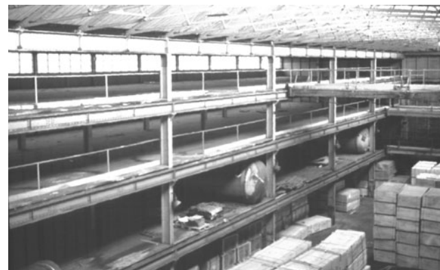
Figure 19. The Boat Store, Sheerness (1858–60), in which stability of the frame is achieved with rigid-jointed cast iron columns and cast and wrought iron beams. (Bill Addis)
